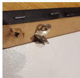
Next - Four of the 12 L shaped brackets that hold the top to the frame had been torn out.
